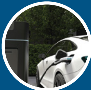
EV- Charge Provision
